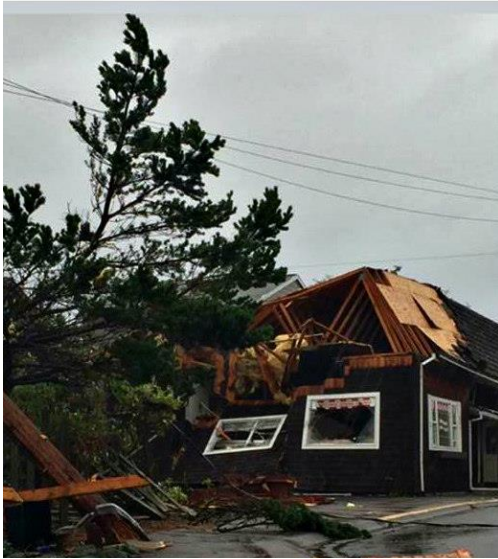
Tillamook County Pioneer, EF-2 tornado damage in downtown Manzanita, OR 14 Oct
